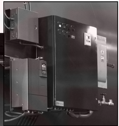
Example of multiple junction box's including: Burner control panel, power disconnect, VFD controller, and junction box, Figure 31c
