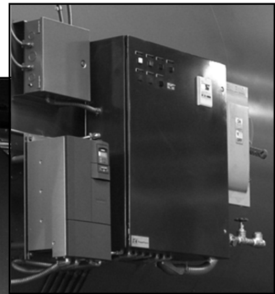
Example of multiple junction box's including: Burner control panel, power disconnect, VFD controller, and junction box, Figure 39c
